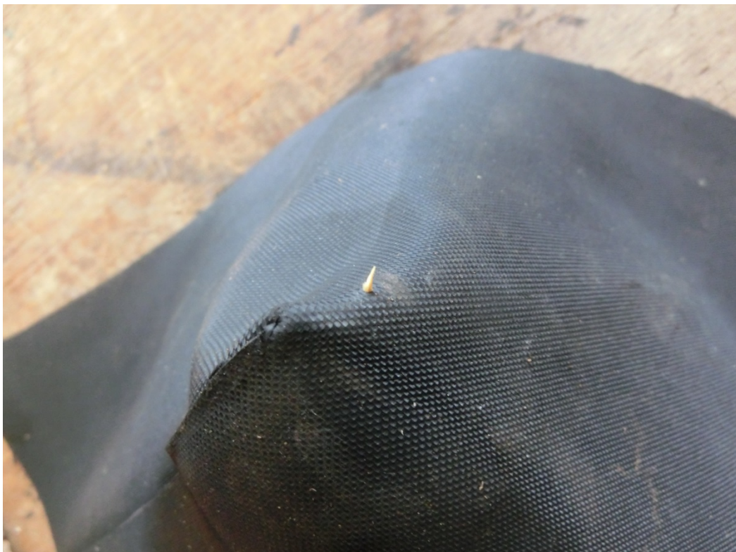
Figure 4: Perforation of the membrane by a rhizome (outer face of the membrane)
